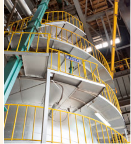
Photo 5: Multiple Hearth Furnace (courtesy: Nomura Kohsan Co., Ltd.)
