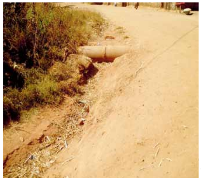
Erosion of road drains.
