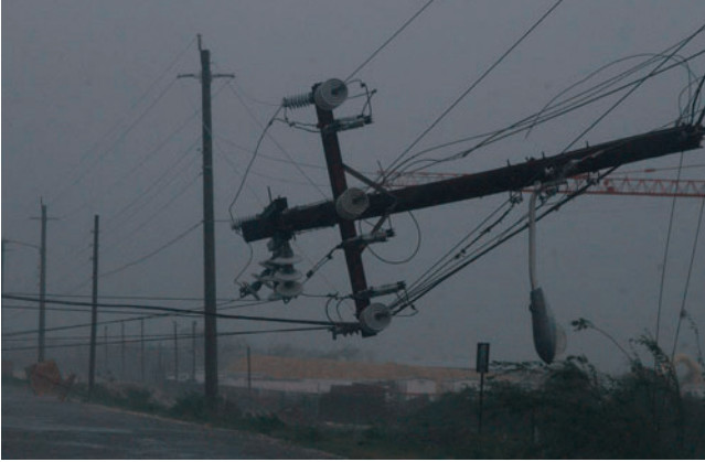
Electrical poles damaged by Hurricane Ivan in Jamaica.
