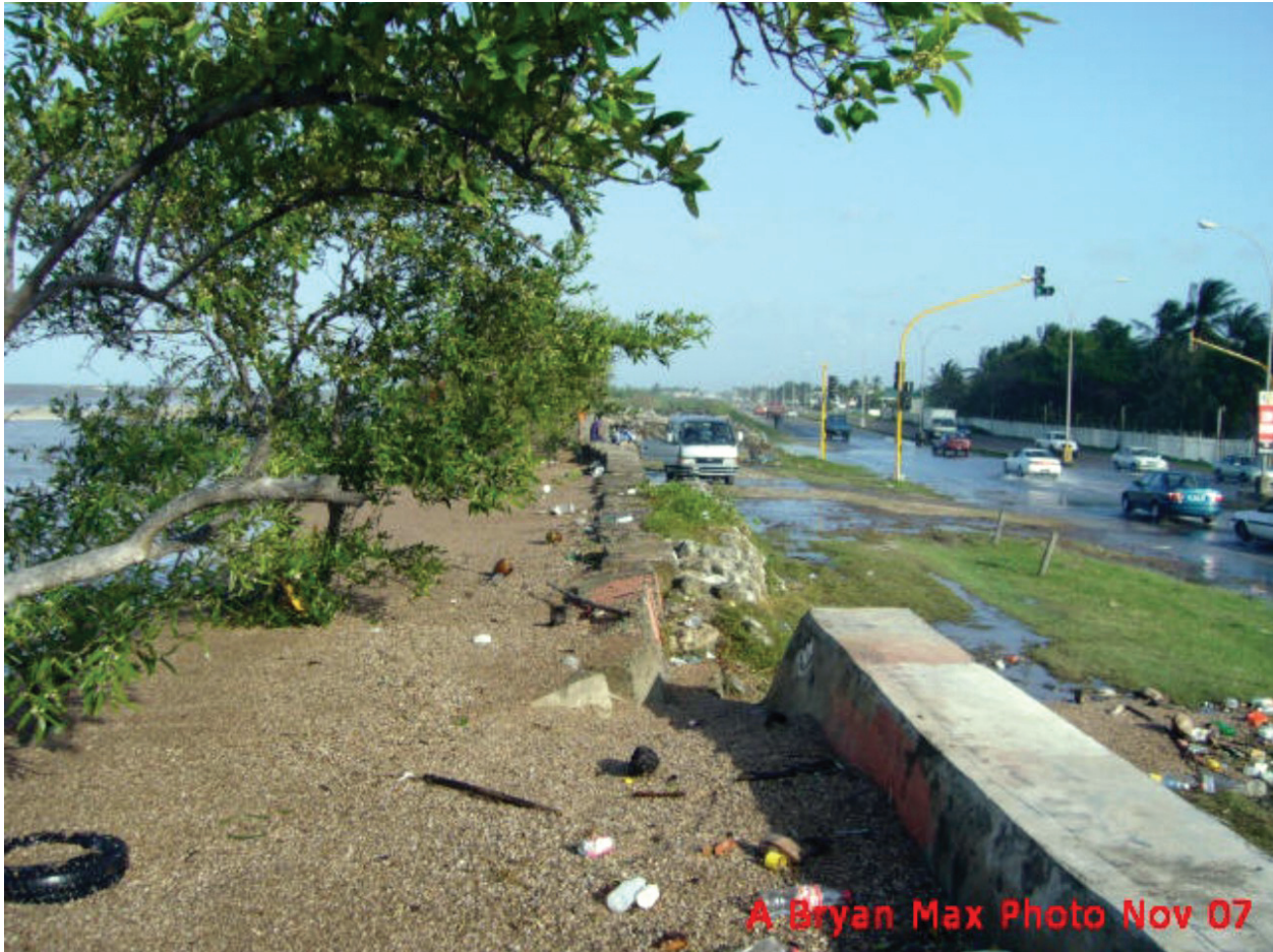
Plate 3.1: Flood Waters Eroding the Sea Defence http://www.bryanmaxx.netfirms.com/may2007/P1000647.JPG
