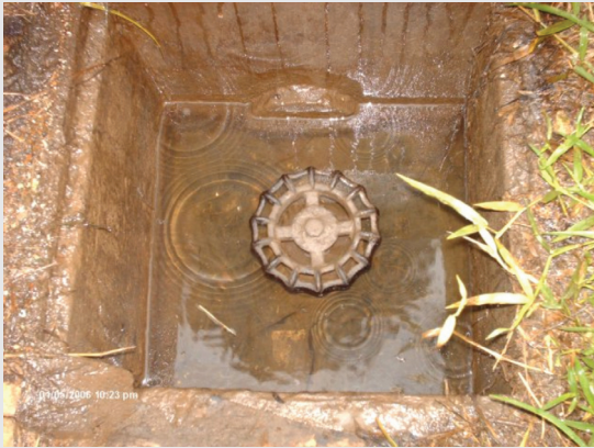
Plate 4.1: Drain Valve for Oil Water Separator Source: Banks DIH
