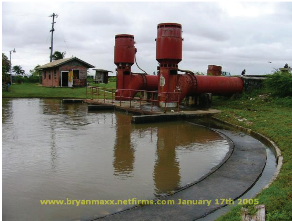
Plate 1.1: Example of Drainage Pumps Installed Along the Coast
