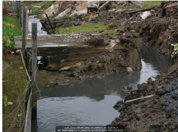
Plate 3.5 Response to blocked drain
