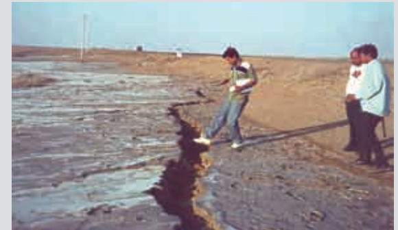
A big tentational crack (approximately 30 cm deep) in a nearby field on Bhuj, Khewda. Salt water had come up to the surface through the crack due to liquefaction. Credit: Ramesh P. Singh/UNEP/Indian Institute of Technology, Kanpur
