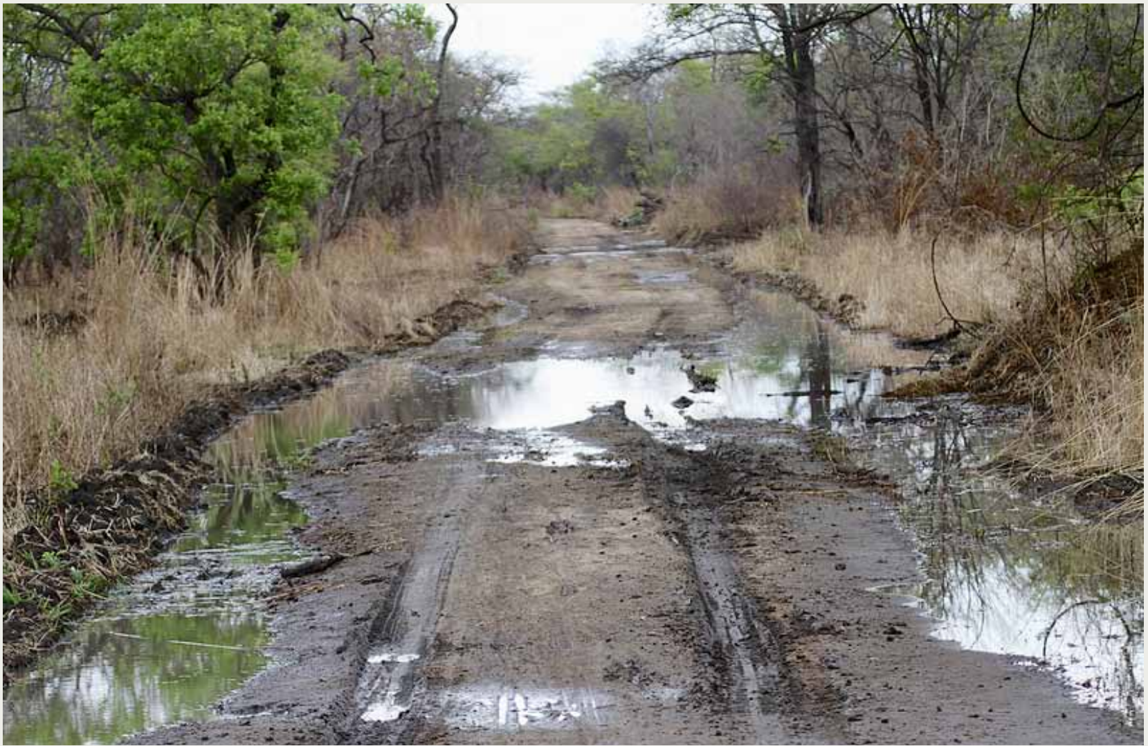
Heavy rainfall episodes can make some roads impassable.
