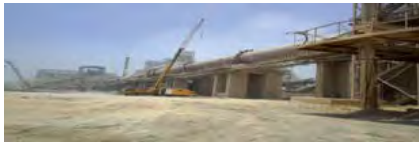
Fig (11-1) Rotary Kiln Line No. (1)
