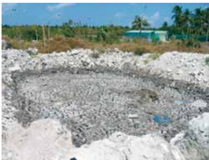
Sludge-drying bed on HD. Kulhudufushi. Credit: E. Spitaler
