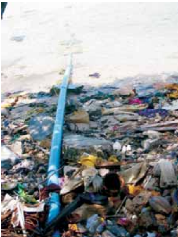
Exposed small-bore sea outfall on K. Vilifushi. Credit: E. Spitaler
