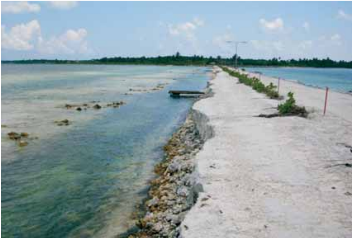
Extensive erosion and scour on western side of the causeway connecting L. Fonadhoo and L. Kaddhoo. Credit: B. Richmond
