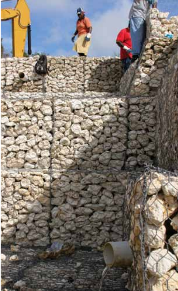
Traditional gabion technology used for road stabilisation programmes in the Scotland District. Photo: Anne Gonzalez
