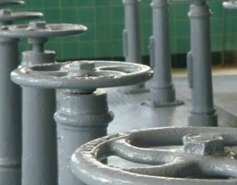
The Belle Pumping Station. Photo: Travis Sinckler
