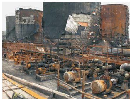
Novi Sad, bomb damage at oil refinery
