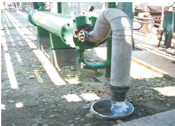
Groundwater remediation, discharge of treated water
