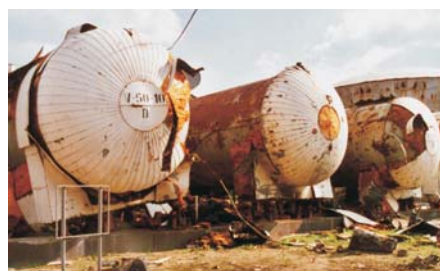
Pancevo, chlorine storage tanks
