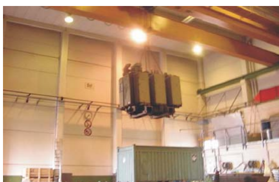
Unloading of damaged PCB-transformer at disposal facility
