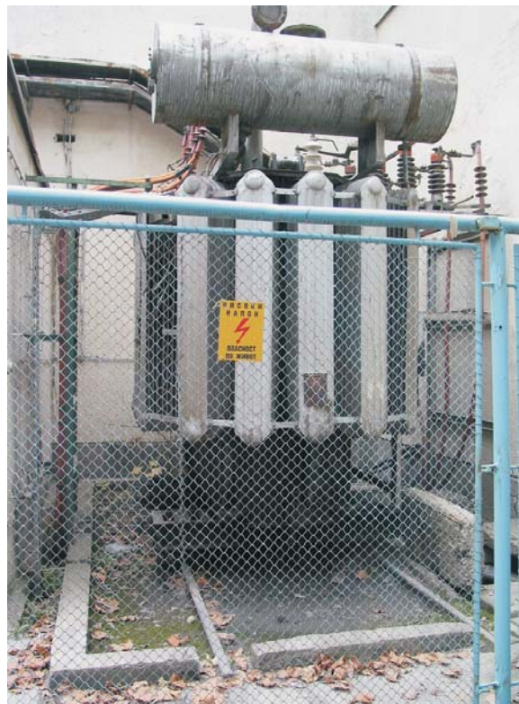
Remediated transformer station at 'Zastava Energetika'
