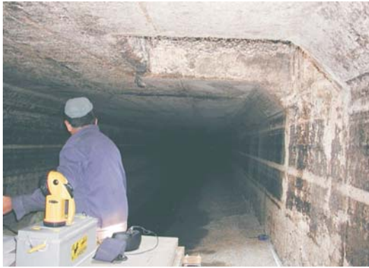
Inside of the collector prior to repair works
