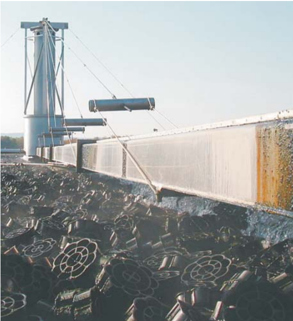
Refurbished trickling filter in operation
