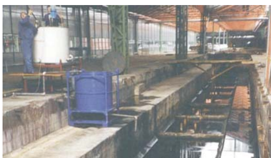
PCB-contaminated wastewater pit in Zastava paint hall
