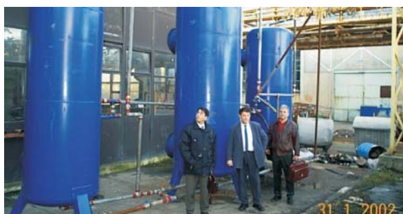
Equipment for treatment of PCB-contaminated wastewater from paint hall pits
