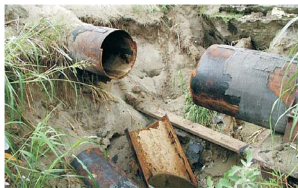
Damaged section of the pipeline from oil refinery
