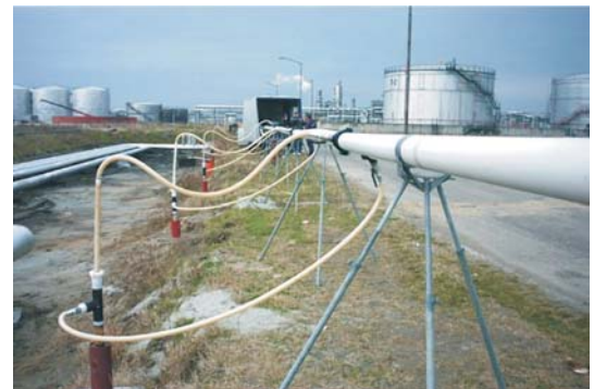
Remediation of free-phase oil overlying the groundwater table at Novi Sad refinery
