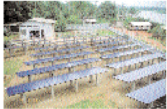
The modular nature of RETs, such as this 50 kW PV array, means the system can grow as power is needed. (Photo: Roger Taylor, courtesy NREL)
