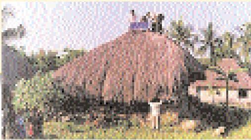
A PV panel, such as this one being installed on the roof of a building, can provide electricity to power lights and small appliances. (Photo: Ullal Harin, courtesy NREL)
