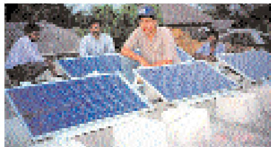
RETs, such as this PV system, can offer a clean leap over fossil fuels in developing countries. (Photo: Jim Welch, courtesy NREL)
