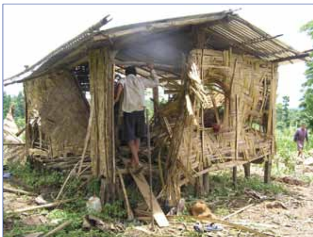
Property damaged by elephant. (PEI Bhutan).
