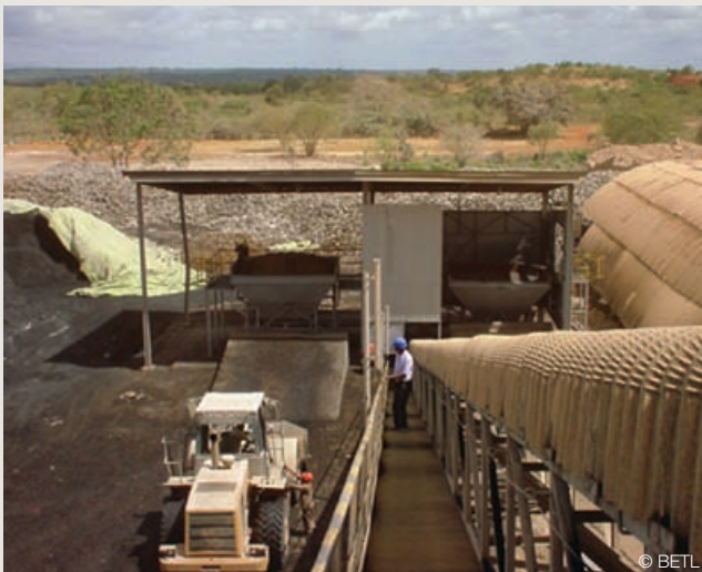
Biomass waste supplied by BETL being loaded to supply energy in cement production.
