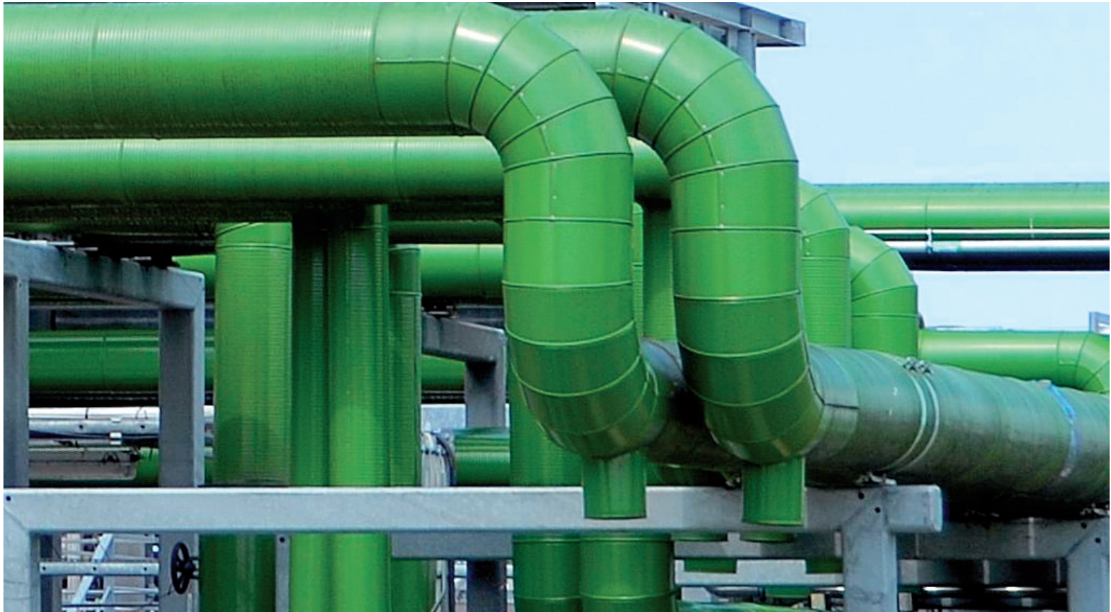
Steam pipes from a power plant and ethanol upgrading facility for reuse at the Kalundborg Symbiosis Industrial zone in Denmark.
