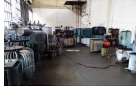
Picture 40: Transformer maintenance area
