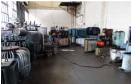
Picture 51: Fire near a substation
