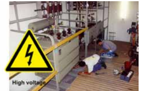
Picture 2: Consider also electric safety precautions
