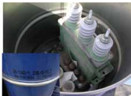
Picture 68: PCB capacitors in steel drum
