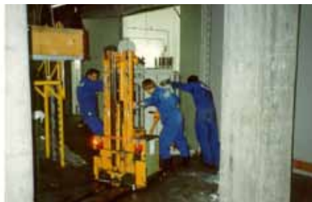
Picture 54: Phase out of an intact PCB transformer
