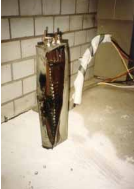
Picture 50: Burst capacitor
