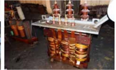
Picture 41: Active transformer part in Albanian workshop
