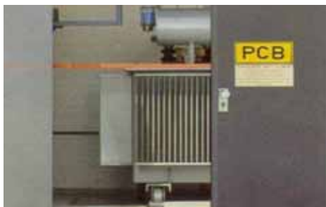
Picture 38: Labelling of a transformer room door
