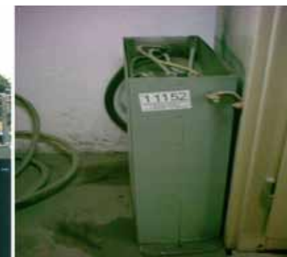
Picture 56: Inventoried and labelled capacitor
