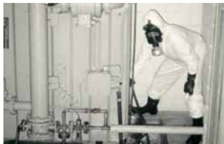
Picture 53: Draining of a PCB transformer
