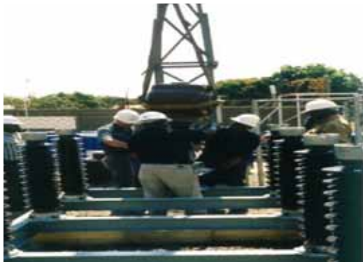
Picture 57: Bad example of packing and storage
