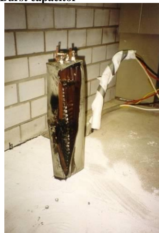
Picture 50: Burst capacitor
