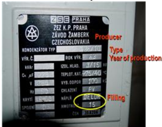
Picture 11: Identification of Capacitor Fluid
