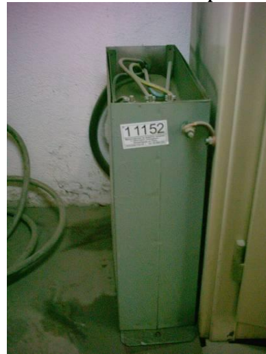
Picture 56: Inventoried and labelled capacitor
