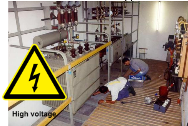
Picture 2: Consider also electric safety precautions
