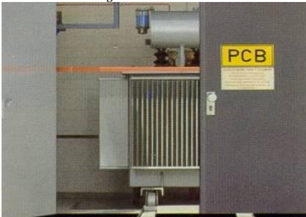
Picture 38: Labelling of a transformer room door
