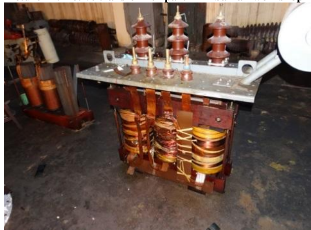
Picture 41: Active transformer part in Albanian workshop
