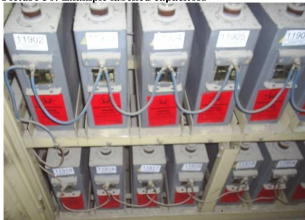
Picture 36: Example labelled capacitors
