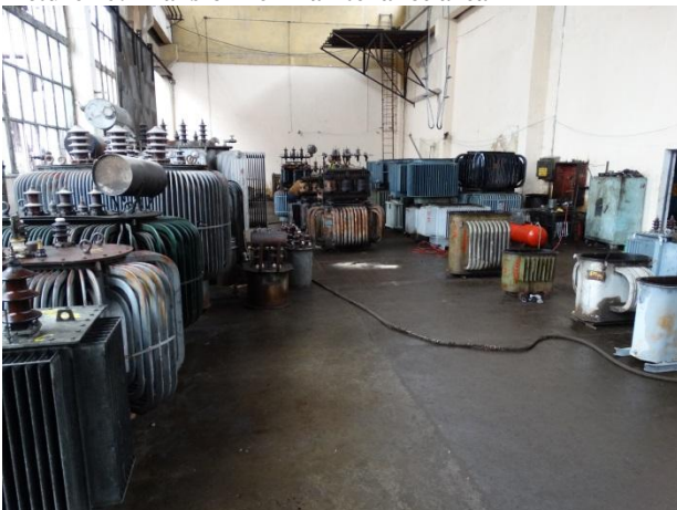
Picture 40: Transformer maintenance area
