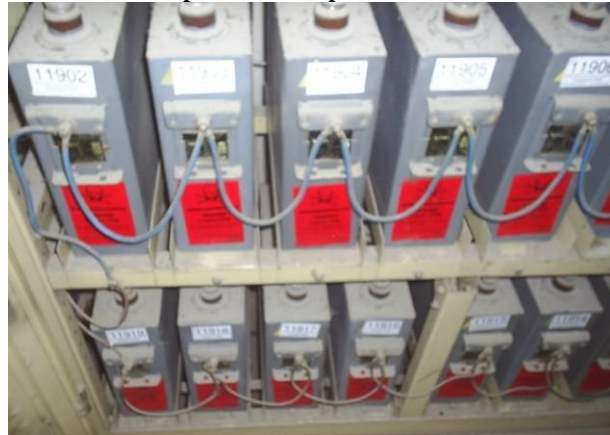
Picture 36: Example labelled capacitors
