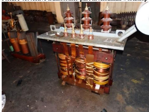
Picture 41: Active transformer part in Albanian workshop
