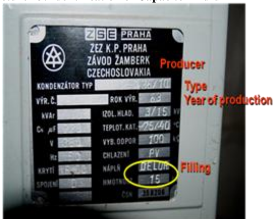
Picture 13: Identification of Capacitor Fluid
