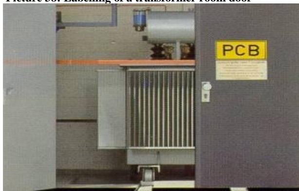
Picture 38: Labelling of a transformer room door
