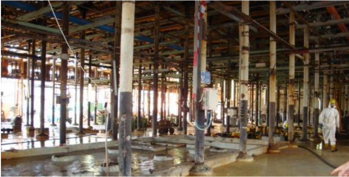
Floor of cell room regularly washed down
