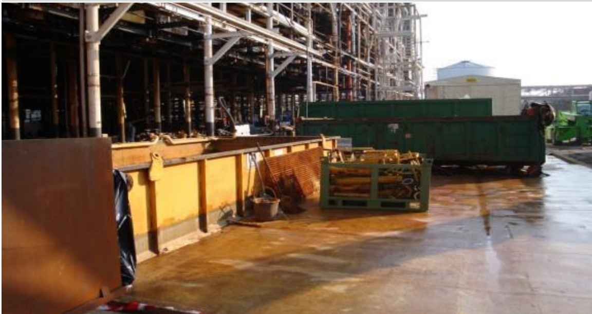
Working area for safe handling of contaminated equipment connected to the Hg effluent treatment unit, regularly washed down with water
