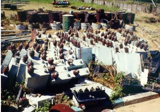
Picture 84: Bad example I (open air storage)
