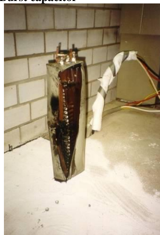
Picture 50: Burst capacitor
