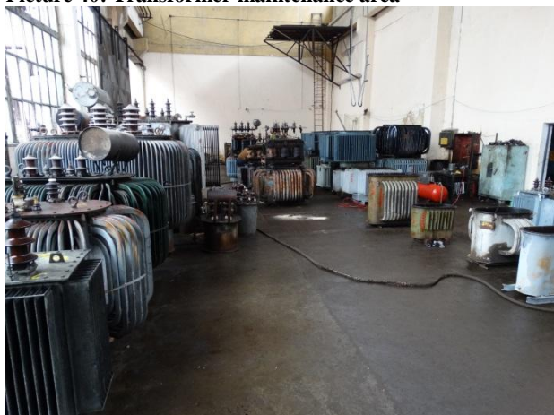
Picture 40: Transformer maintenance area
