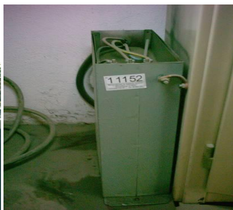
Picture 56: Inventoried and labelled capacitor
