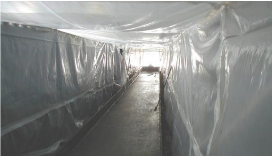
Cell confinement (connected to the air treatment unit)
