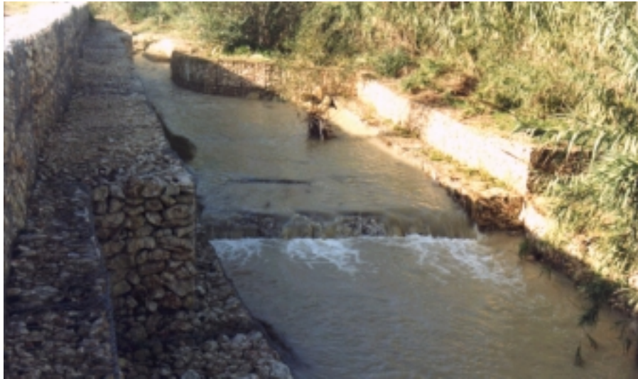
Plate 2: Adoption of a gabion system to avoid soil and rubble wall erosion
