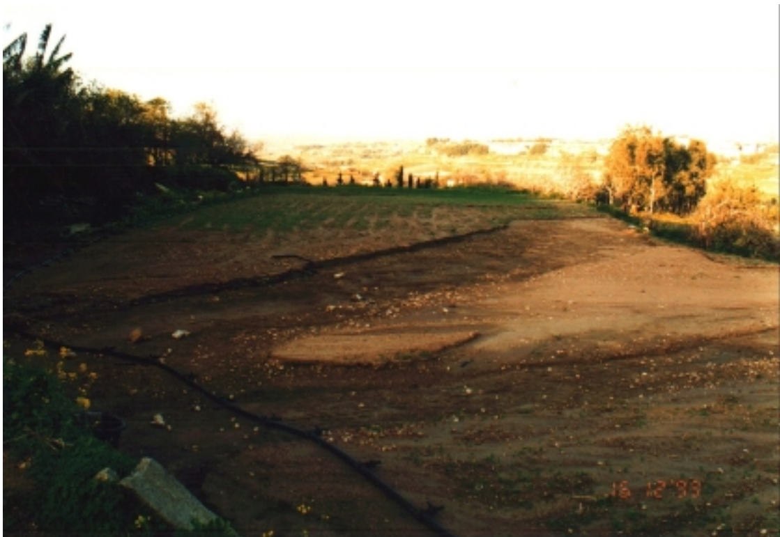
Plate VI. 25. Following the construction of a peripheral road at Dingli, storm waters were channelled onto the fields located down slope and about 20cm topsoil was carried away (November, 1999).
