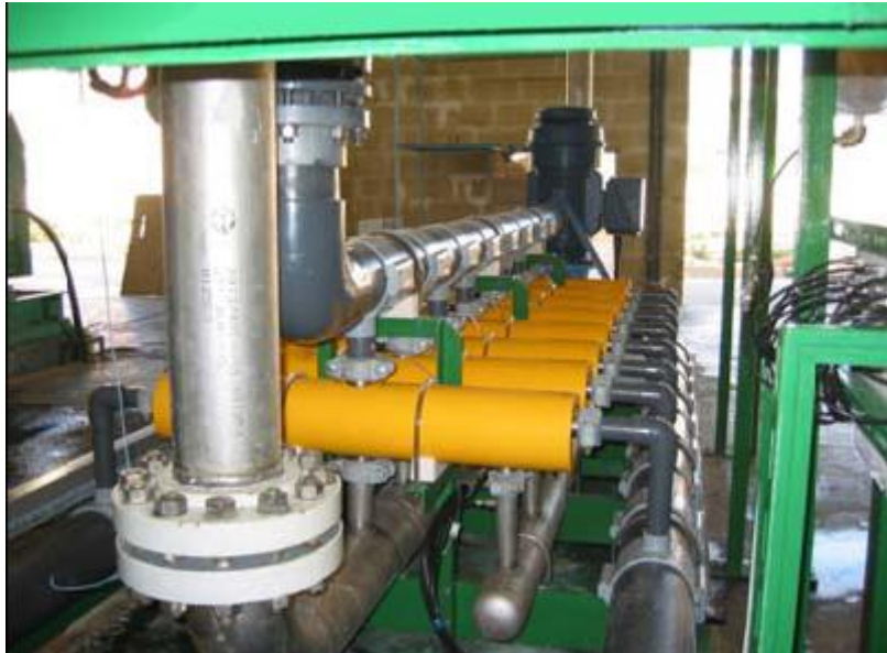
Figure 5 Pressure Exchangers at Lapsi R.O. Plant
