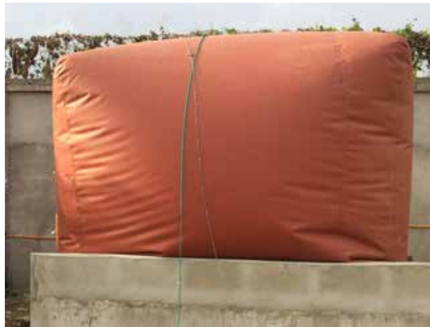
Part of the biogas facility at the learning institution Photo | SUITCH Africa Green
