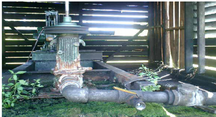
Borehole overhead mechanical pump in Tonga.
