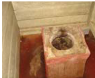
School sanitation improvement project in the Driver's River Watershed – Before the intervention
