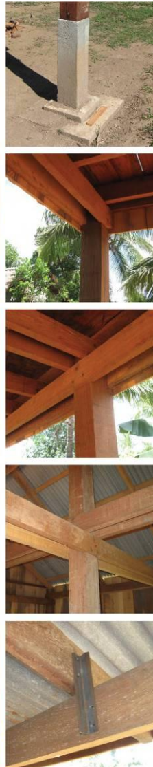
Improved cyclone proof solution
