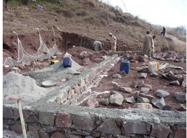
Fishing net is wrapped underneath stone foundation
