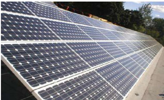
Photovoltaic panels, used to produce electricity
