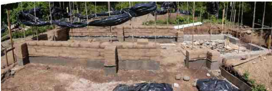
Adobe walls under construction, including plinth, pilasters, vertical reinforcement and plastic rain-covers.
