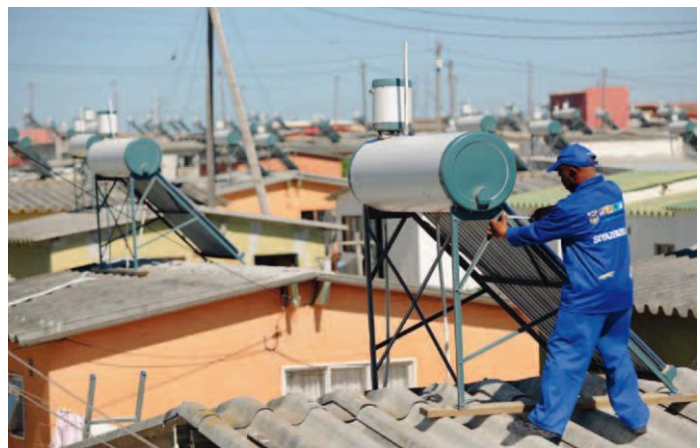
Solar panels for hot-water production 37
