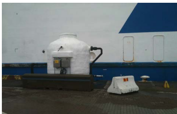
Sewage collection in Trelleborg port (Sweden) (Photo credits: Clean Baltic Sea Shipping)
