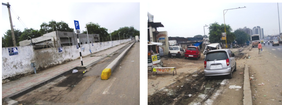
Figure 4.12 (Left) Autorickshaw parking planned at entry to bicycle track (Right) State of bicycle tracks after rains
