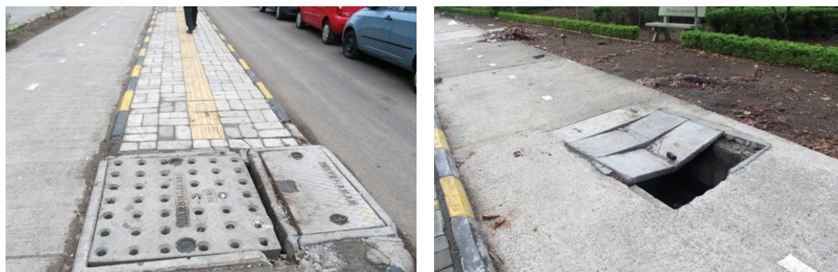
Figure 3.26 Inspection chambers on NMT lanes
