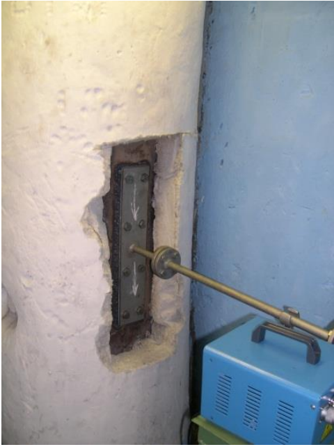
Figure 6. ACI lance inserted into the gas duct.
