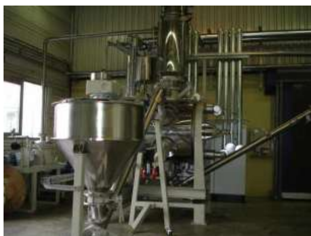
Figure 5 DELA stabilization plant (Source: DELA GmbH)
