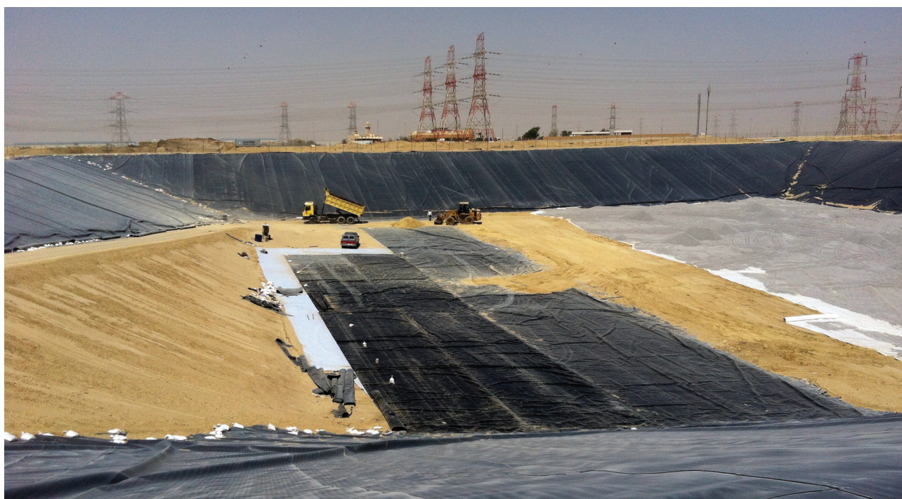
Hazardous waste landfill under construction in Kuwait (Source: Courtesy of National Cleaning Company, Kuwait)
