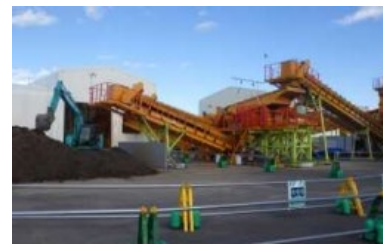
Crushing and sorting facility at a temporary site in Naraha, Fukushima Source: MOEJ
