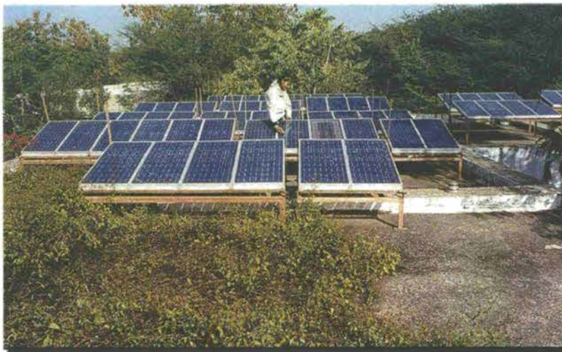
Solar panels provide lighting and power the telephone exchange
