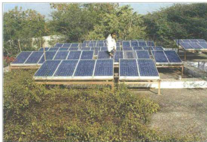
Solar panels provide lighting and power the telephone exchange
