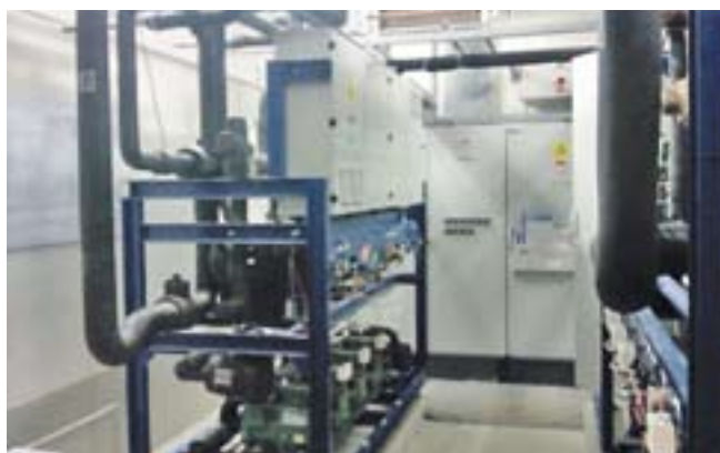
Kaufland CO 2 /HFC-134a cascade system installed in Croatian shopping center in Vukovar
