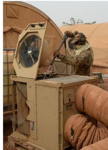
IMAGE: A HEATING, VENTILATION AND AIR-CONDITIONING (HVAC) UNIT GETS A CLEANING AT AN AIR FORCE BASE IN NIGERIA. View more > CREDIT: JIMMIE PIKE/US AIR FORCE
