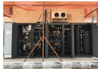
The transcritical CO 2 refrigeration system being installed at the Al Salam military supermarket in Amman, Jordan
