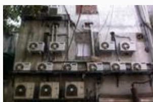
Air conditioner units in India. NRDC
