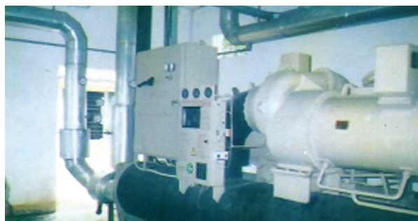
CFC-11 Chiller at Nha Trang Textile Factory
