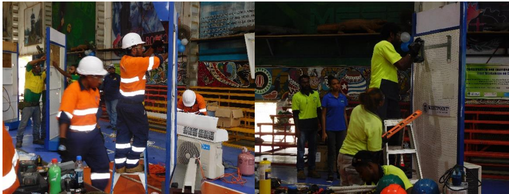
Figure 5: Industry Teams South Pacific Air-conditioning (Left) and ABCO PNG Ltd (right) in action during the installation category of the competition.
