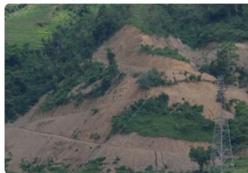
EB road at Bhainse, Makwanpur, showing ruthless stripping of the natural environment
