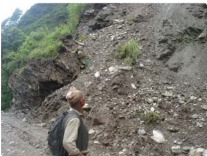
Common landslide events in EB VDC roads
