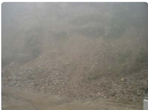
Landslides begin as soon as the EB road section is entered, Mude–Melung road, Dolakha district
