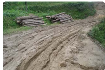
Road damaged by local neglect
