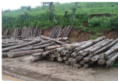
Soil dumped into road to create timber storage space
