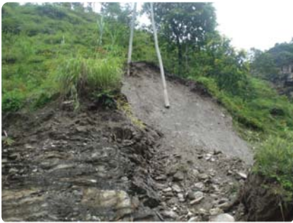
Landslides do not even spare electrical poles
