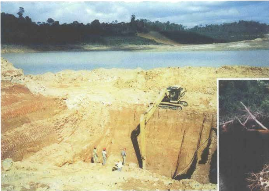
Left: In the aftermath of the accident, extensive forensic work was carried out on a cross-section of the dam to determine reasons for the failure.
