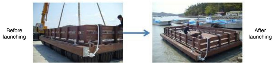
Figure 4. A floating receptacle before and after launching into port.
