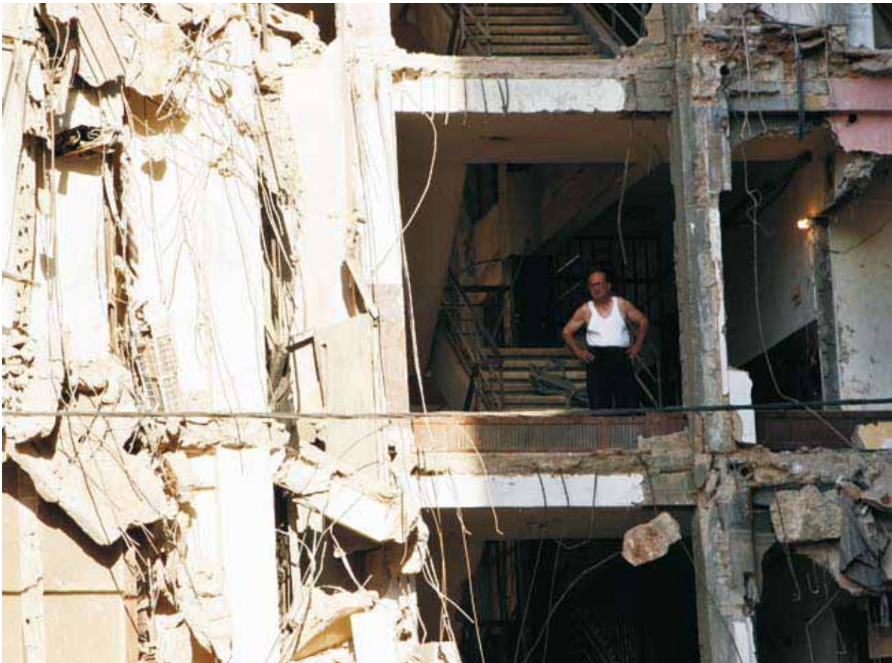
A severely damaged building in the southern suburbs of Beirut
