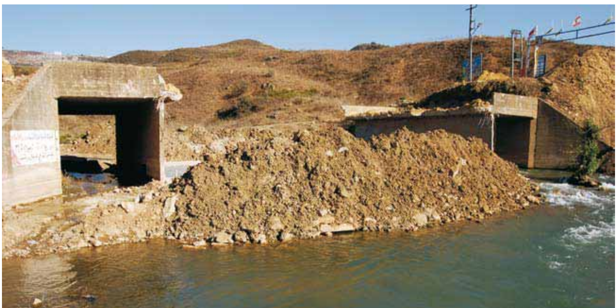
Debris from destroyed bridges, such as this one on the Litani River, could lead to flooding in the rainy season
