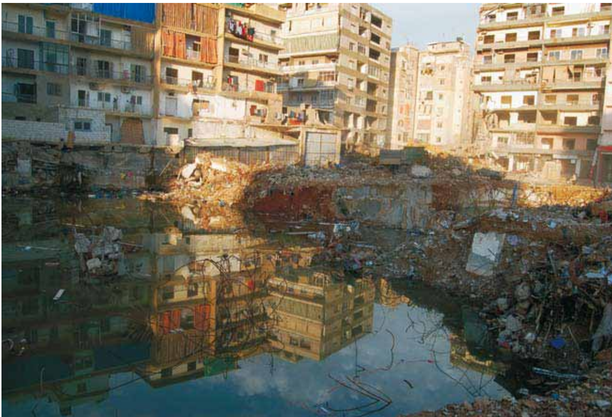
Water trapped in the excavation site of a destroyed building in Security Square, in Haret Hreik
