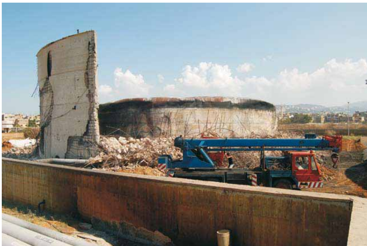
The concrete base of the damaged fuel storage tank at Beirut's airport was being demolished
