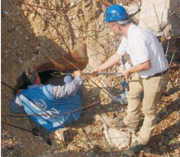
UNEP experts inspect a damaged fuel tank
