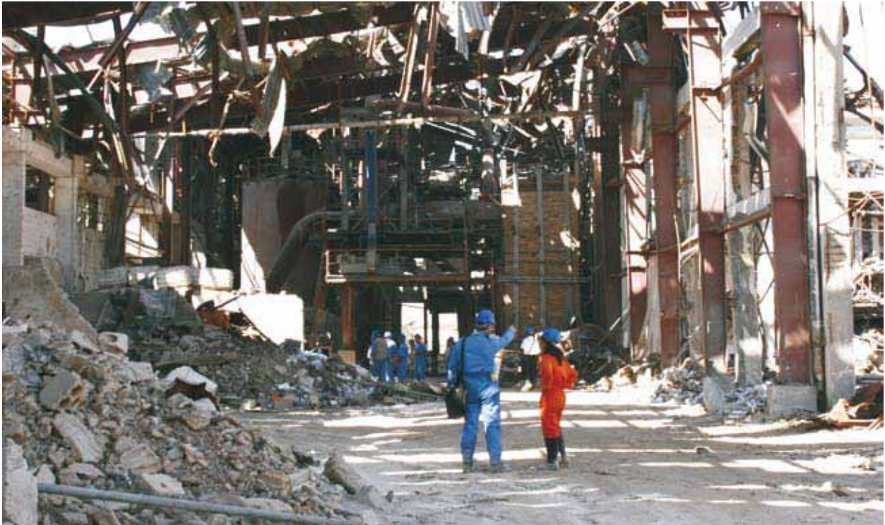
UNEP and local experts inspect a damaged glass factory in Zahleh
