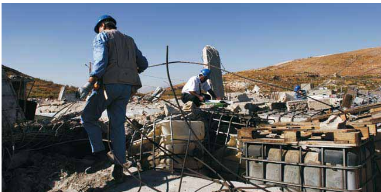
UNEP inspects the damaged structure of the textile factory
