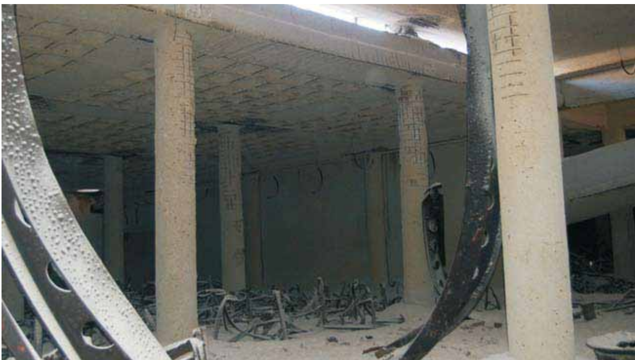
The Transmed Industry in Beirut shows typical damage from the impact of a 'bunker buster' bomb
