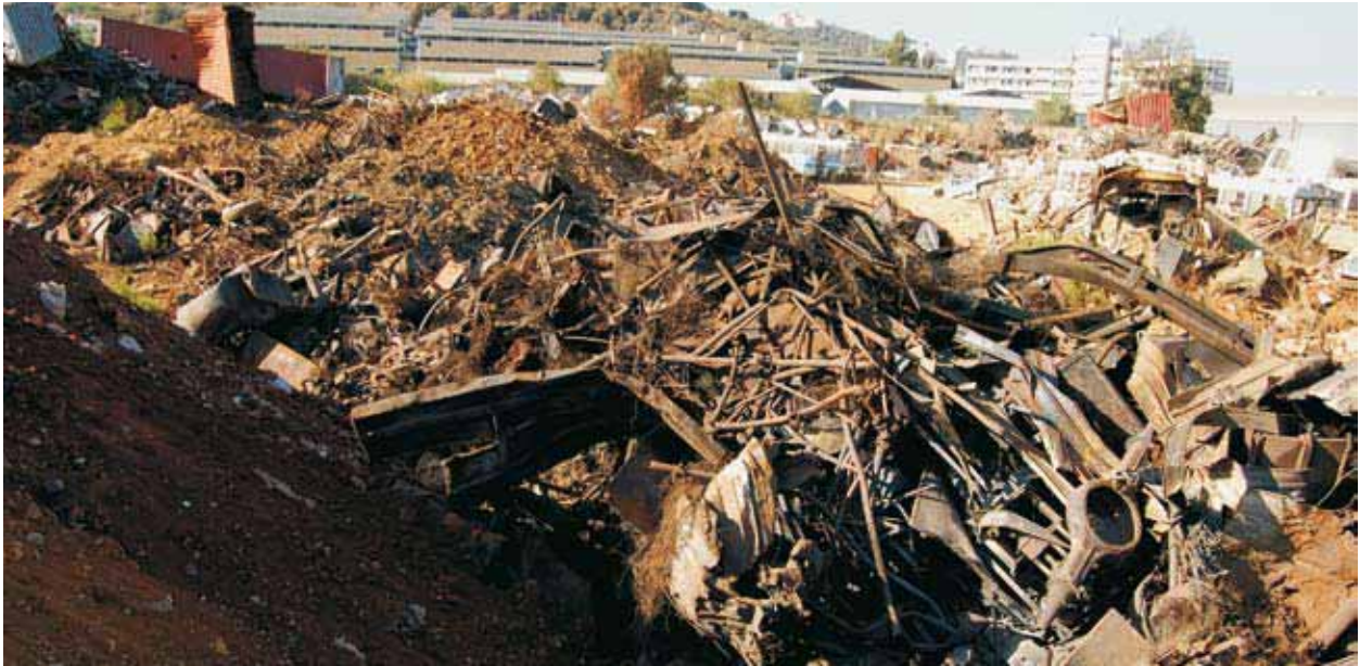
Demolition waste at Lamartine Food Industry requires disposal
