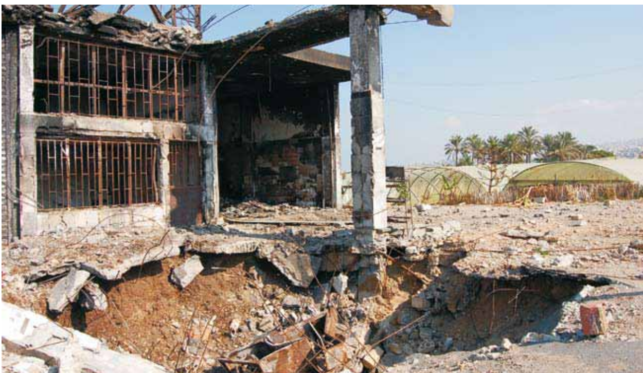
The severely damaged Saida fuel station with bomb crater in the foreground
