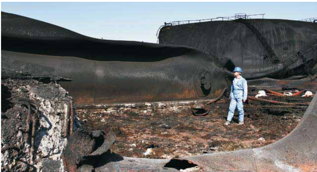
UNEP expert assessing damaged fuel storage tanks at Jiyeh power plant
