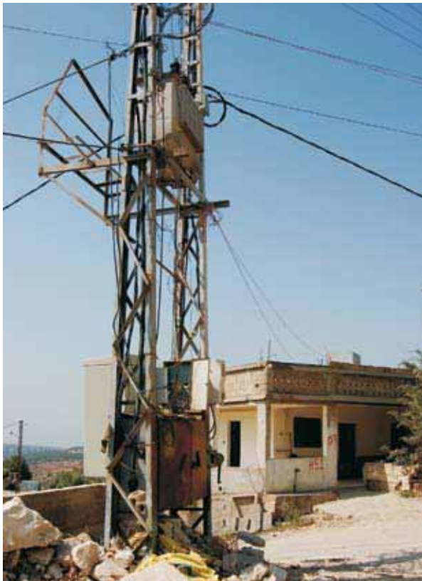
The new transformer that has replaced the one damaged in the conflict
