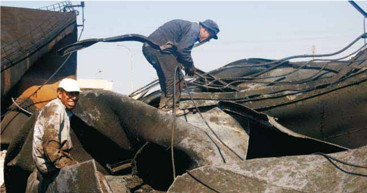
Dismantling of the fuel storage tanks was ongoing at the time of assessment. The complete absence of personal protective equipment for staff was a concern
