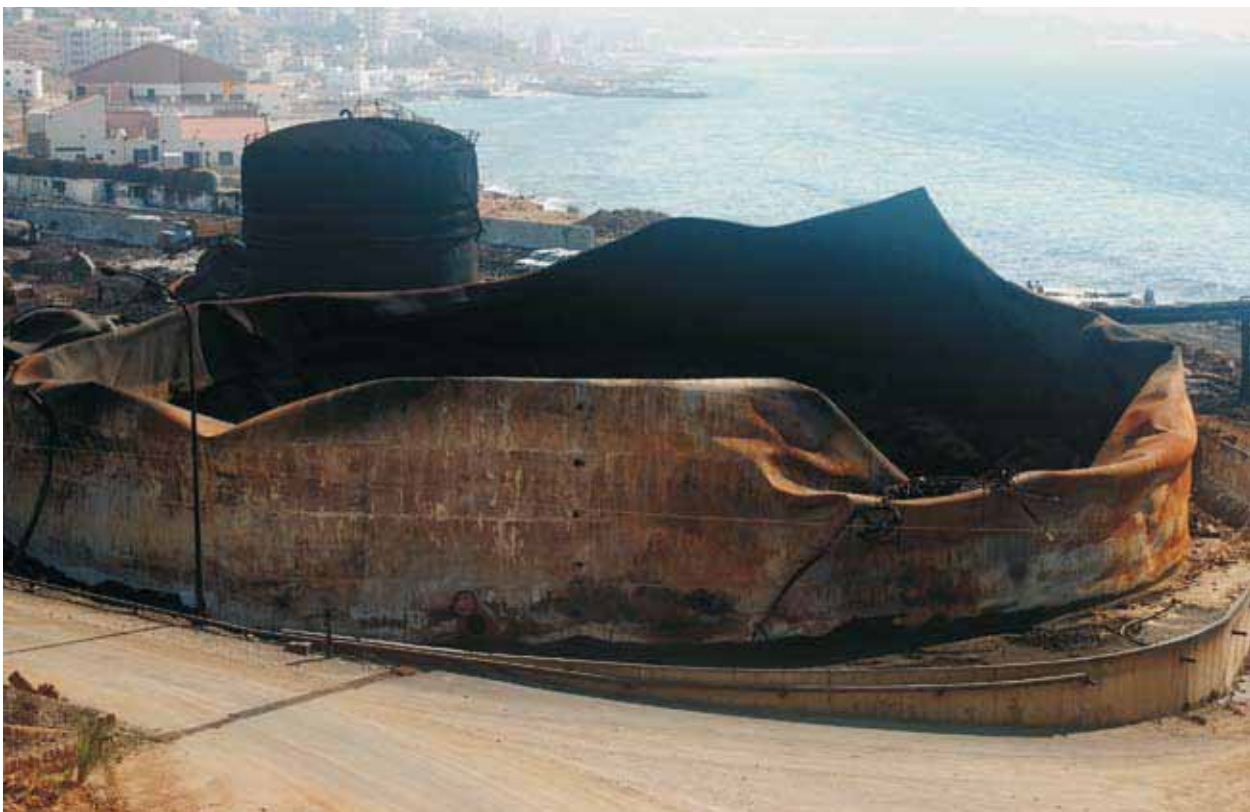
The remains of the fuel storage tanks at the Jiyeh power plant
