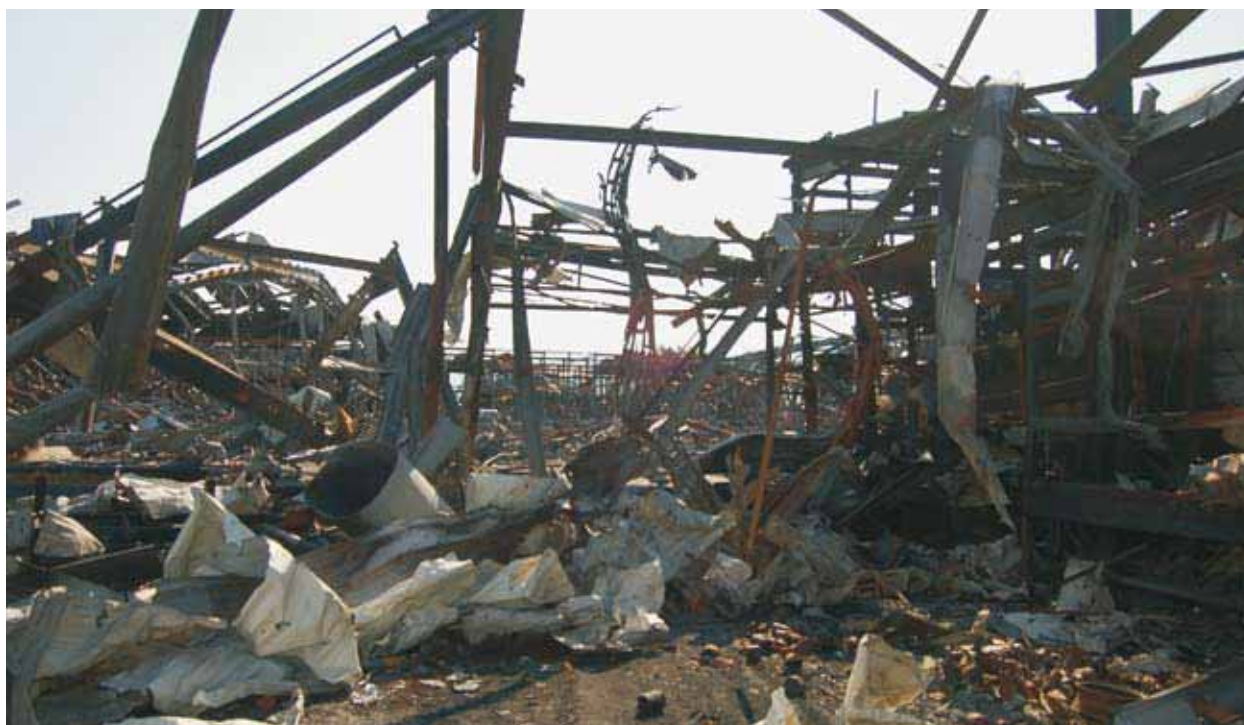
The Transmed facility was extensively damaged during the conflict
