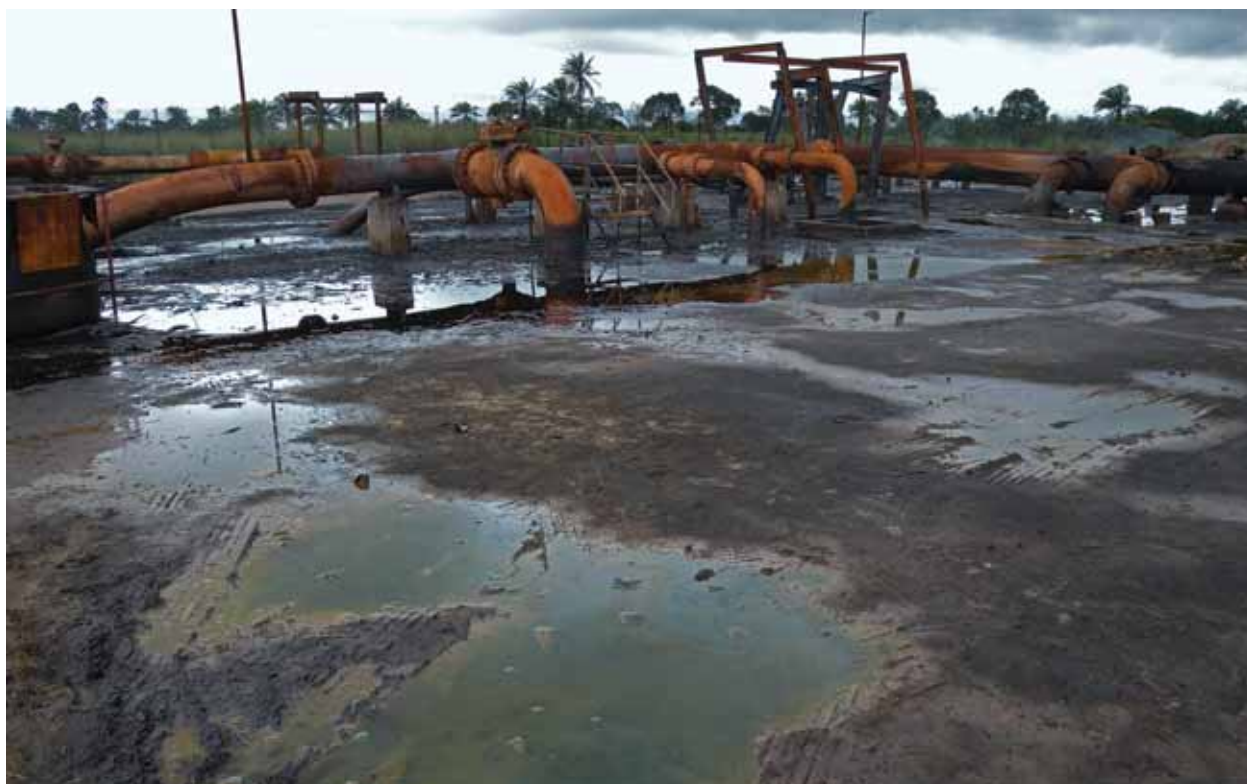
A view of the Bomu flow station (K-Dere, Gokana LGA)
