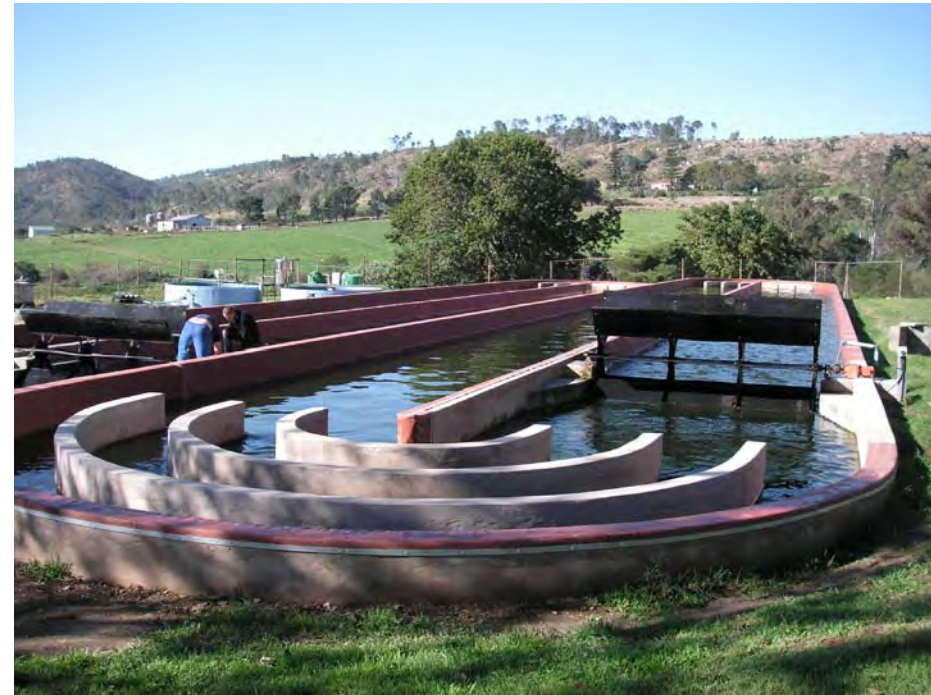
Innovative wastewater treatment at Grahamstown, South Africa (Photo courtesy of Peter Scheren)
