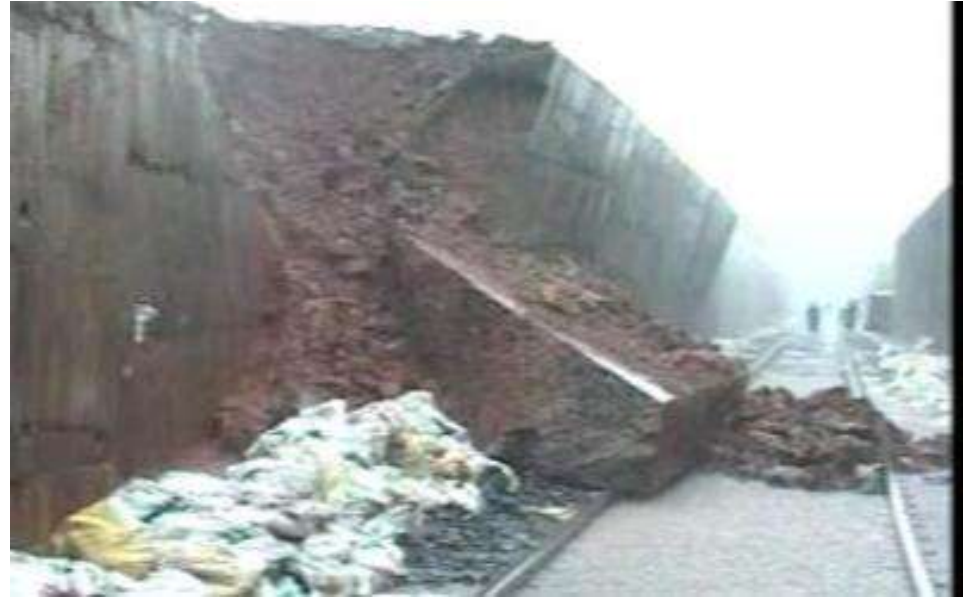
The collapse of retaining wall between Nivasar and Ratnagiri stations in Konkan Railway
