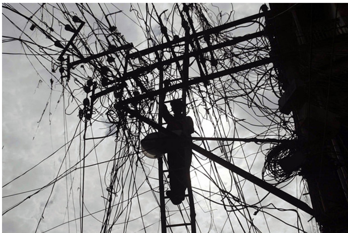
Figure 2 An electrical linesman repairs cables in Allahabad, India. Illegal subsidiary wires are tangled into main cables (WSI, 2009)
