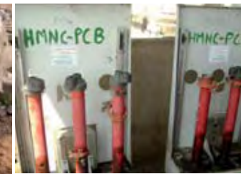
Circuit breakers containing non-contaminated mineral oil
