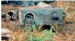
Obsolete stocks of PCB equipment have not been appropriately inventoried yet
