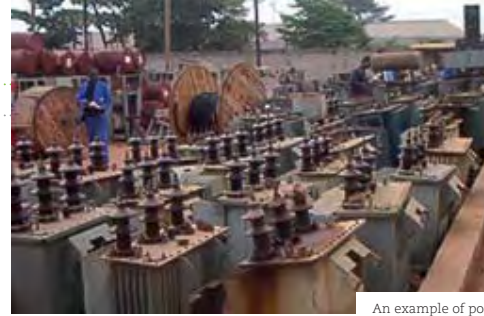
An example of poor storage practice
