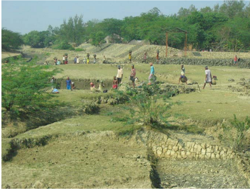
Fig. 3.2: Villagers are building a drainage channel and dykes to regulate yearly recurring monsoonal floods in the lower parts of the Ganges delta, West-Bengal (Photo: Irina Overeem).
