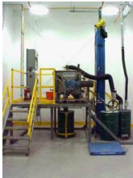
Figure 6 ADA Technology Mercury Treatment Skid (Source: ADA Technologies, Inc.)
