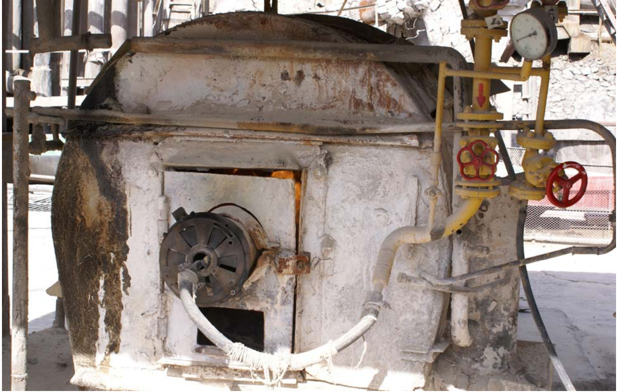
Figure 21 Natural gas burner
